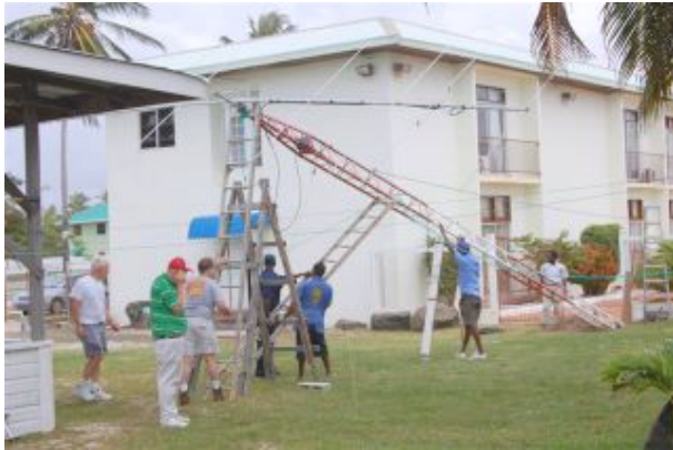
Antenna on Tower, propped up by a ladder
